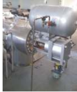
Globe Valve With Pneumatic Actuator for Turbine Protection TGM - CITROSUCO
