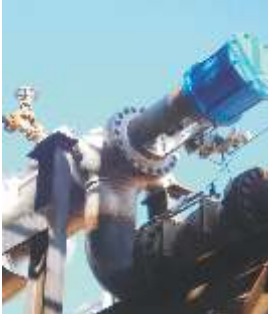
Steam Conditioning Valve USINA COLORADO
